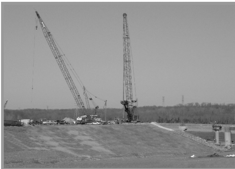
Work is progressing on the relocation of US 62 and the Paducah & Louisville RR to accommodate the expansion of lock facilities at Kentucky Dam. The relocation will see the construction of both highway and railroad bridges. The base for the highway and rail is well underway on the west bank of the Tennessee River. Photo of the construction site was made by Ron Stubblefield.
